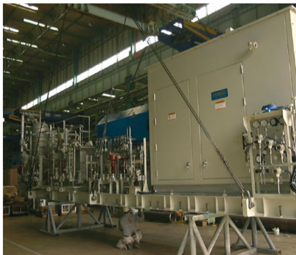
Figure 4. Oil free screw gas compressor for refinery offgas service.
